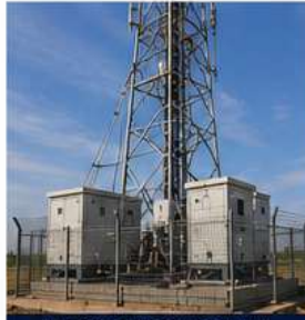
TELECOM SITE DEVELOPMENT Complete site development with equipment shelters and fencing.
