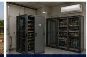
EQUIPMENT ROOM / SHELTER Construction of equipment shelters and telecom rooms.
