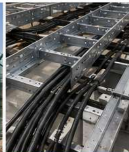
14 CABLE MANAGEMENT Cable tray installation, proper routing, labeling and management.
