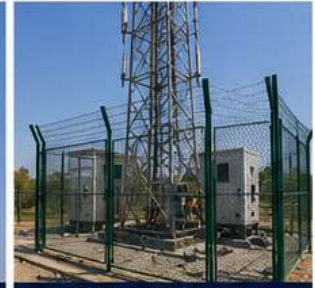
SITE FENCING & SECURITY Perimeter fencing, gates and security systems for telecom sites.
