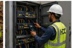
STRUCTURED CABLING Structured cabling for voice, data and communication systems.
